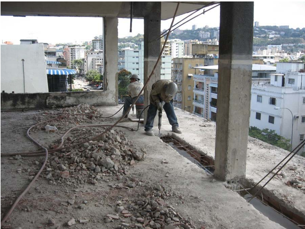
Fig 4: Partial concrete removal for placing new beams using low energy chipping hammers
