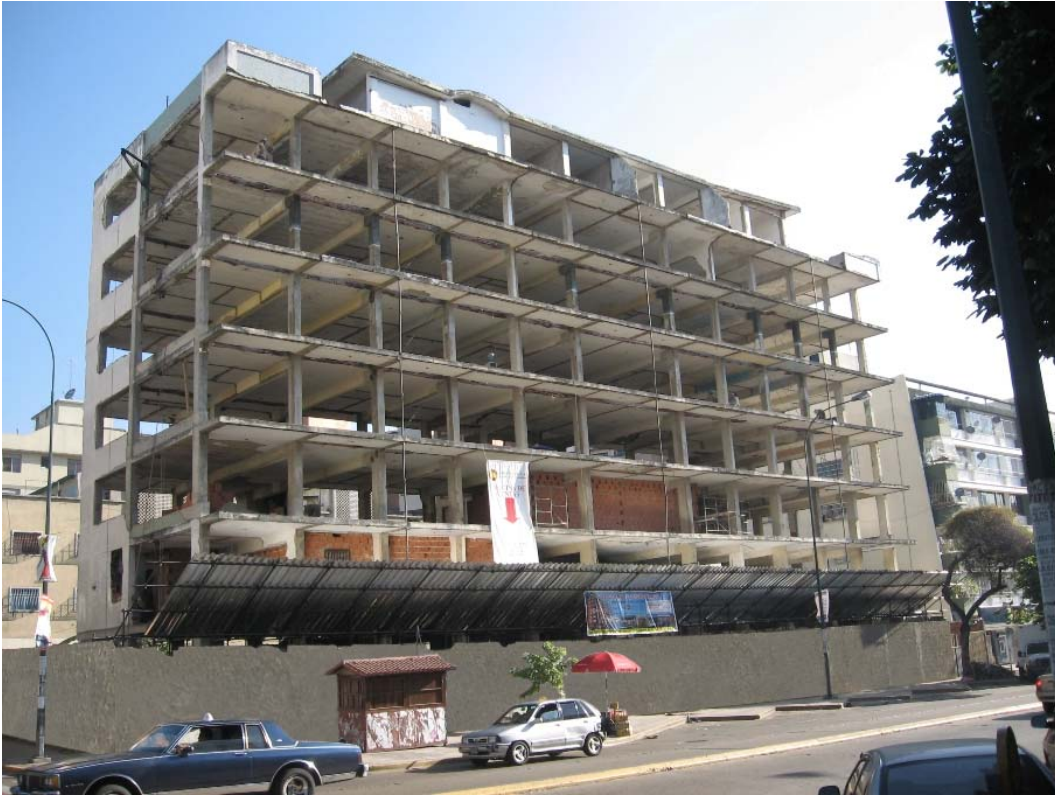
Fig. 1: Building before retrofitting Concrete frames in transverse direction and absence of beams in longitudinal direction
